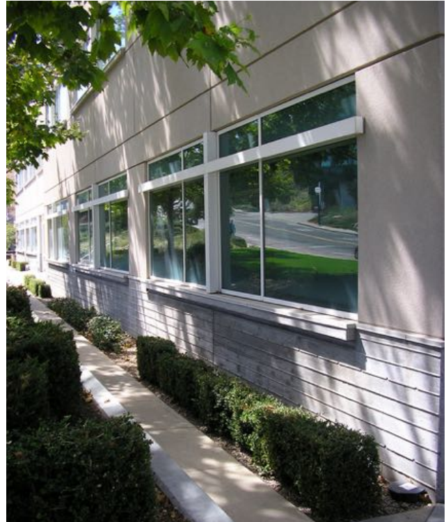
Use of landscaping and formwork ribs in concrete walls to emphasize horizontal orientation of base walls.
