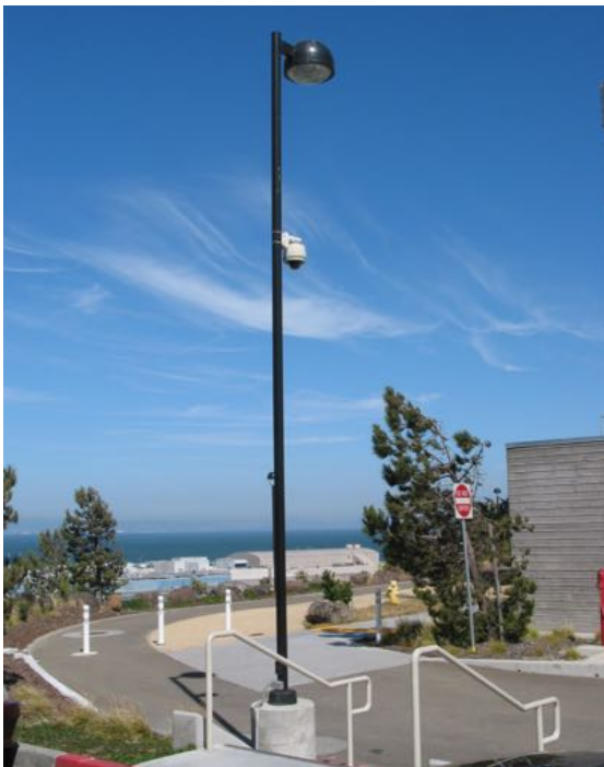
Lighting fixture at parking lot.
