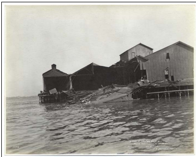
Partial collapse of the Western Creameries wharf due to damage from the teredo worm, November 9, 1920 (Source: H. B. Homer Photo/ California State Library)
